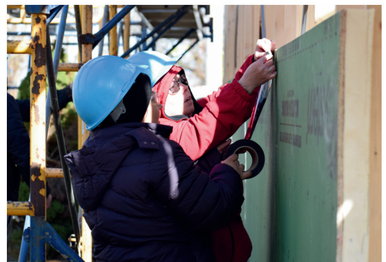
A volunteer helps a partner family member apply sheathing tape to the wall's insulation.
